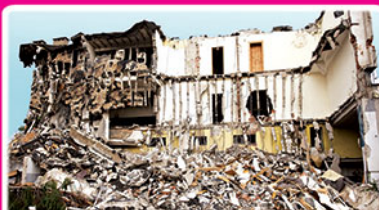
STRUCTURAL COLLAPSE (Building collapse)
