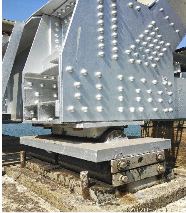
Figure 5. Steel roller type bearing
