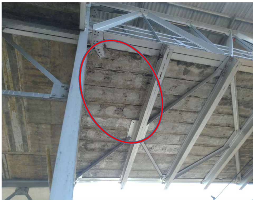
Figure 7. Bottom bracings missing in the second span
