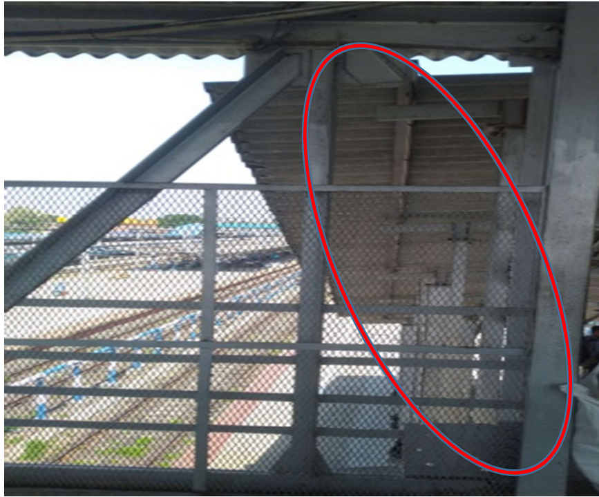
Figure 8. Diagonal member absent in the second span
