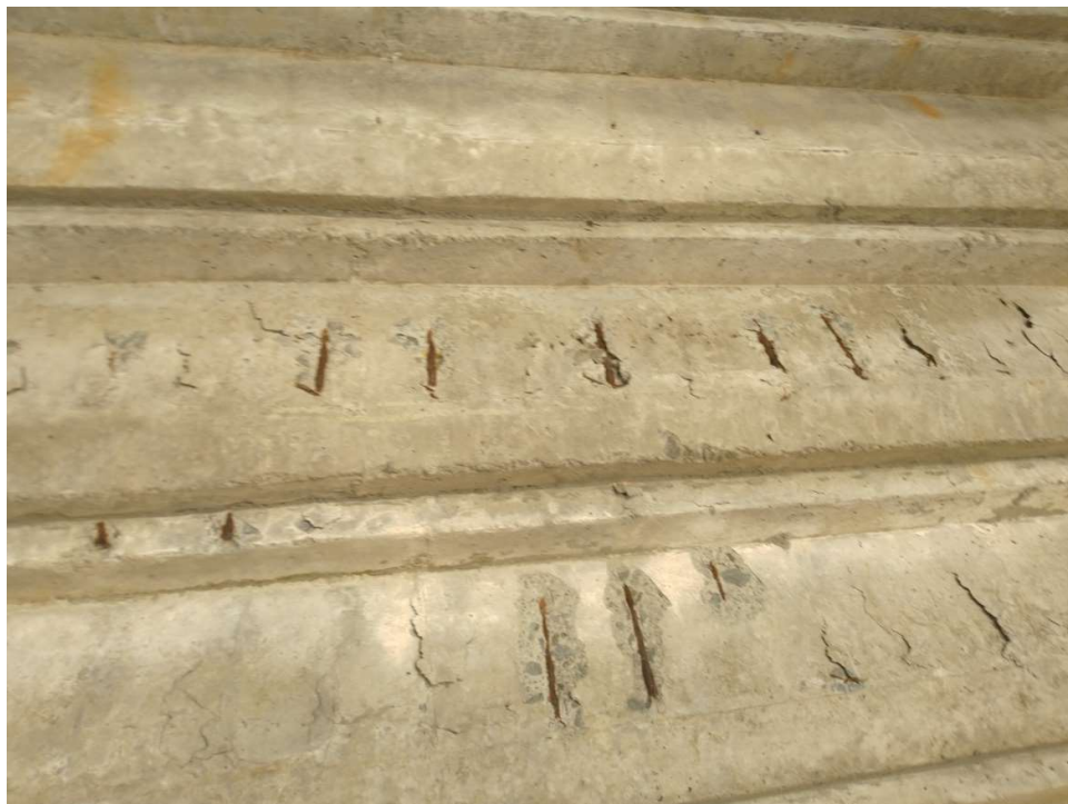
Figure 6. Spalling of concrete at stair slabs
