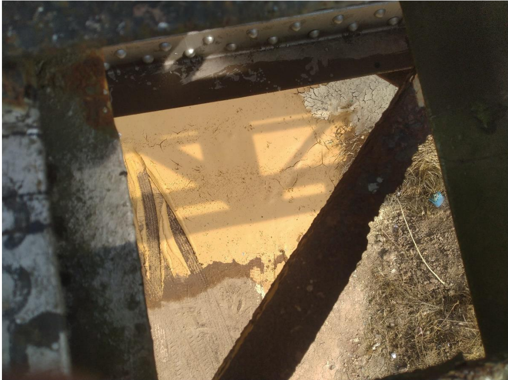
Figure 13. Corrosion in bottom bracing
