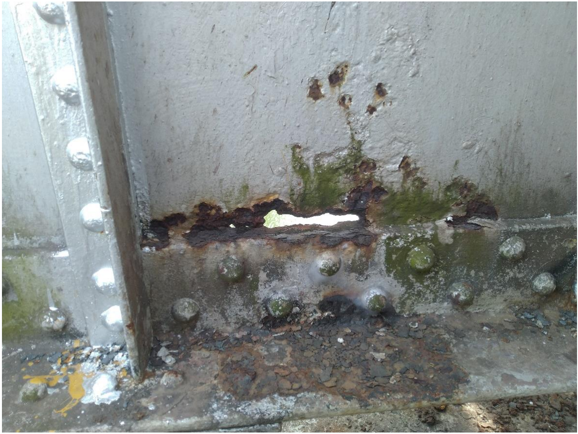
Figure 10. Corrosion in bottom flange main beam
