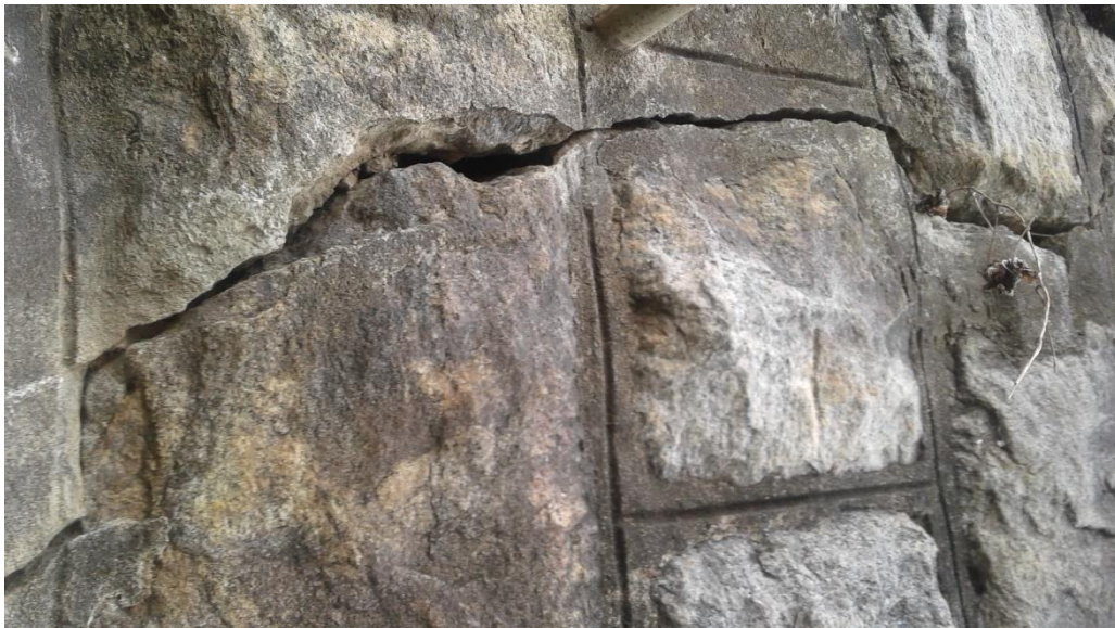
Figure 17. Cracks in the abutment
