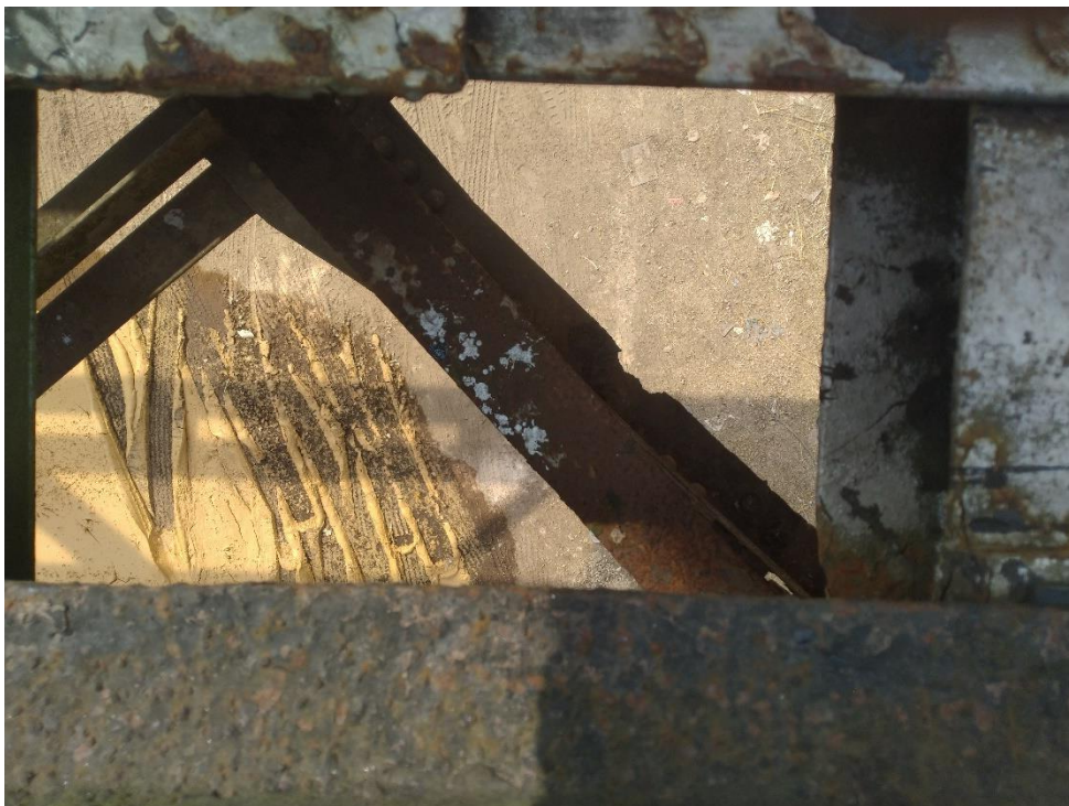
Figure 12. Loss of material in bottom bracing
