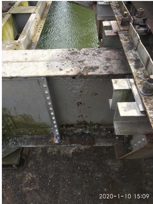
Figure 11. Corrosion in main beam
