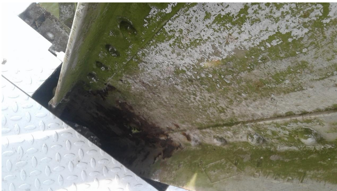
Figure 15. Corrosion in the vertical
