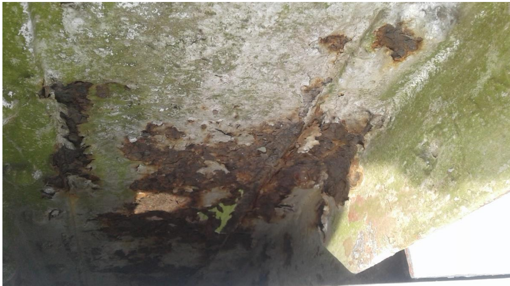
Figure 14. Corrosion in the bottom of verticals
