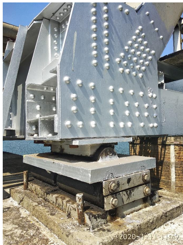
Figure 3. Steel roller type bearing
