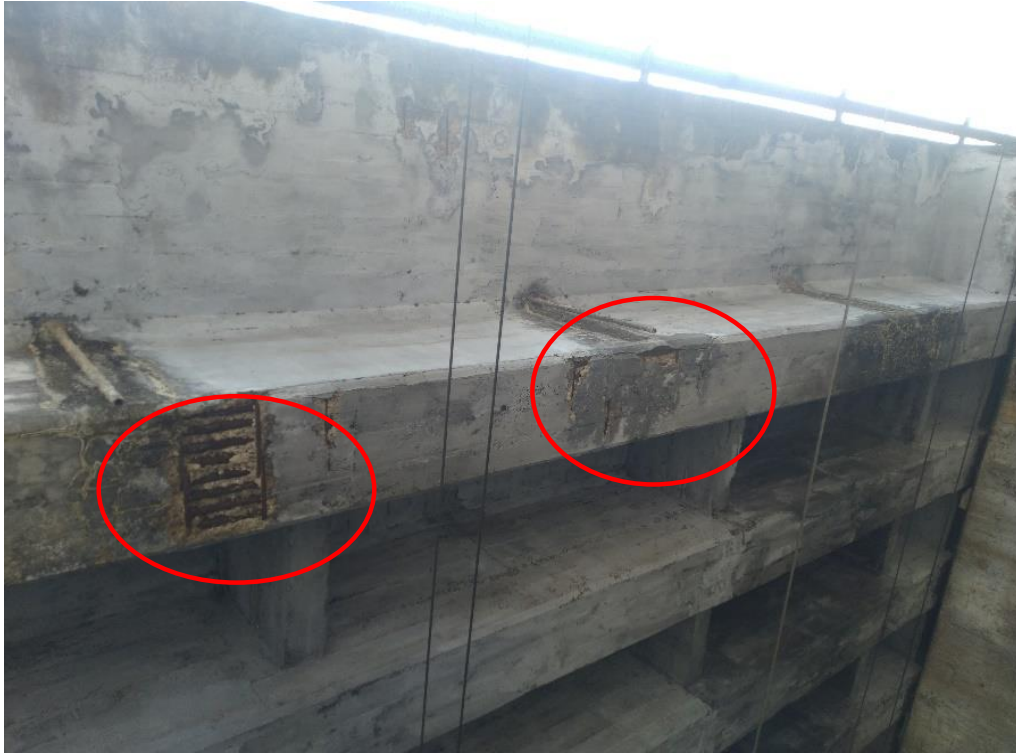
Figure 5. Concrete cover is spalled and reinforcement is exposed at the mid span of end main girder at Calicut side
