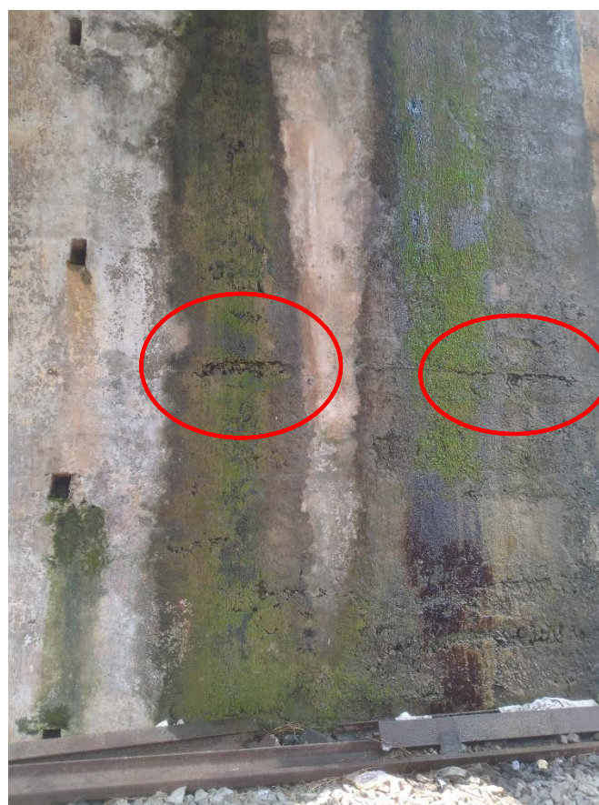
Figure 8. Spalling of concrete at abutment at eastern side
