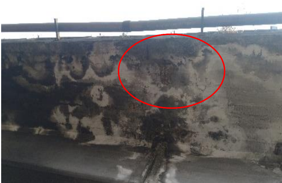
Figure 7. Concrete is spalled and rebar is exposed at bottom of the deck slab at Calicut side
