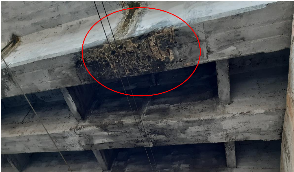
Figure 6. Concrete cover is spalled and reinforcement is exposed at near the support of end main girder at Calicut side
