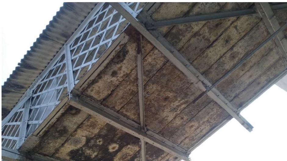
Figure 8. Corrosion of bottom laterals
