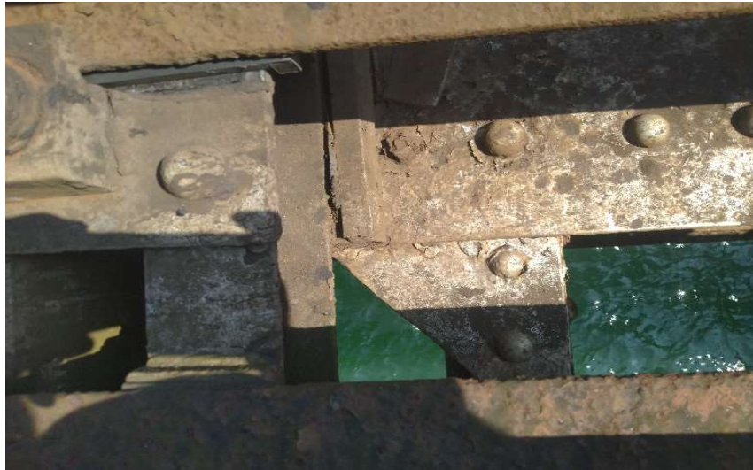
Figure 7. Severe corrosion in rivets
