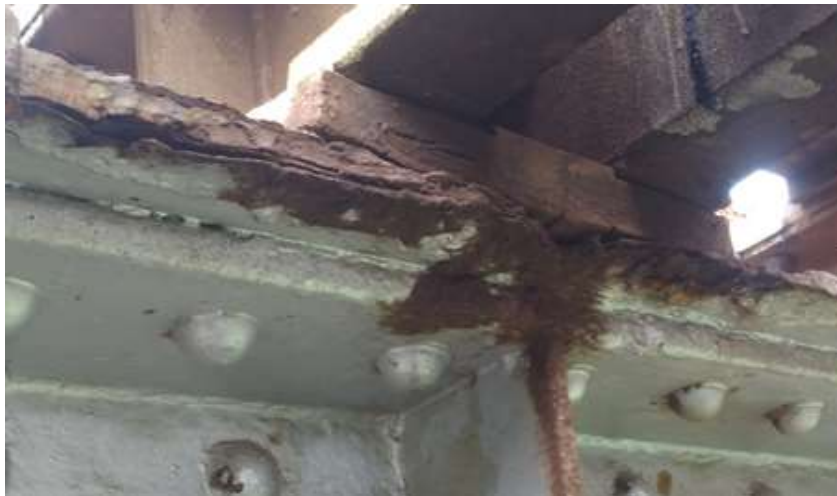
Figure 8. Corrosion in top flange under rail sleepers
