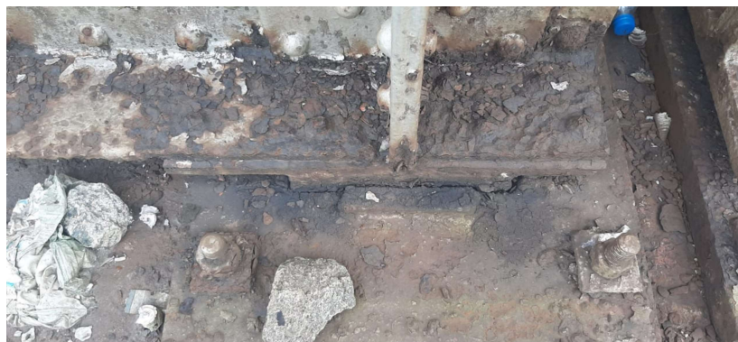
Figure 6. Corrosion of bottom flange over base plate
