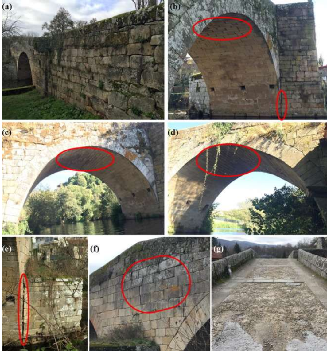
Figure 10: (a) abutment (b) buttress (c) stone deterioration at the crown of arch (d) in-plane deformations of arch and stone deterioration at the crown (e) cutwater (f) out-of-plane deformations and cracks at the spandrel wall (g) damaged pathway.
