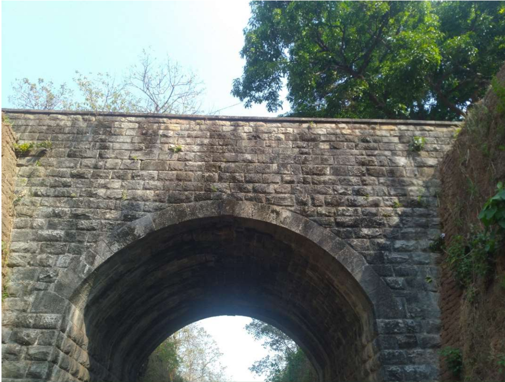
Figure 5. Vegetation growth in backfill near the bridge
