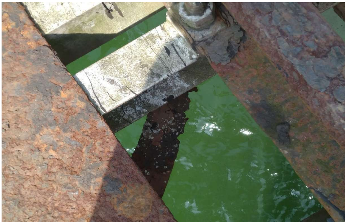
Figure 8. Pitting and material loss in the horizontal bracings
