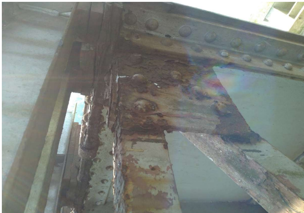
Figure 5. Corrosion and material loss in the gusset plate and rivets
