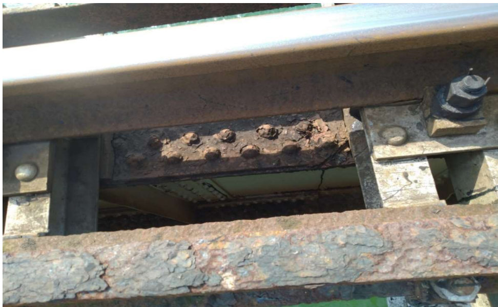
Figure 11. Corrosion and material loss in the rivet heads
