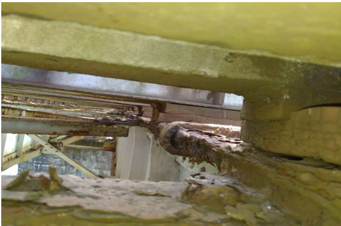
Figure 6. Corrosion and material loss in the top flange
