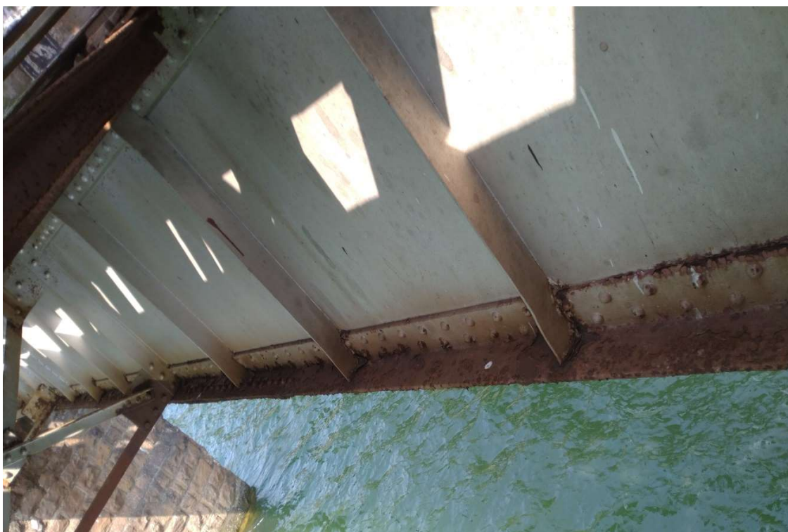
Figure 7. Corrosion in the connecting angle
