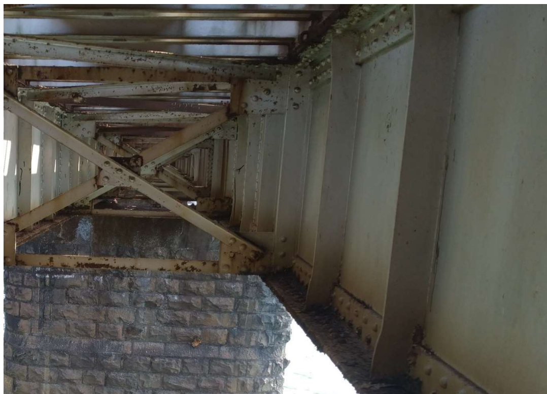
Figure 9. Corrosion and material loss in the cross-bracing elements
