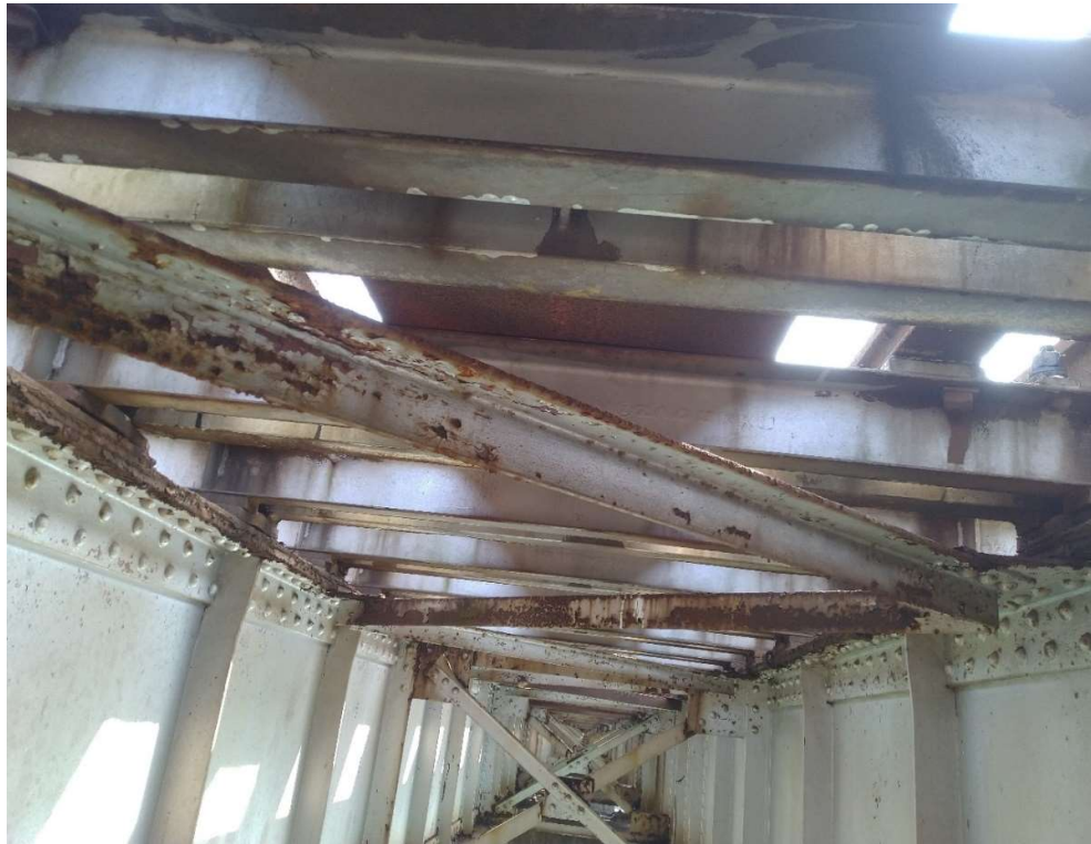
Figure 10. Corrosion and material loss in the horizontal bracing
