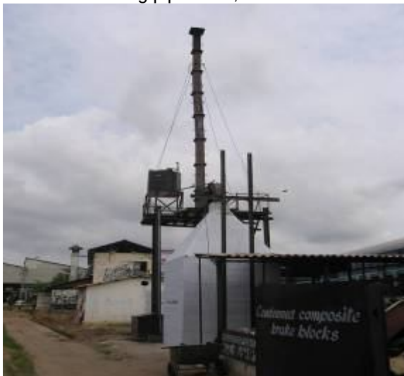
Incinerator after fitment of cooling system
