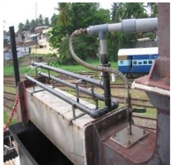
External cooling system
